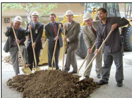
Participants at the ground breaking turn dirt to celebrate Trade-Tech College's first parking structure. From Left to Right: Frank Harris, ASO president at Trade-Tech College in 1952; Greg Fischer, deputy for L.A. City Councilmember Jan Perry; Michael D. Waxman, vice president for the Board of Trustees for the L.A. Community College District; Larry Eisenberg, executive director of Facilities Planning and Development for the L.A. Community College District; Dr. Tom Harris, interim president at Trade-Tech College; Trade-Tech College's ASO President Ethan Burrall.
