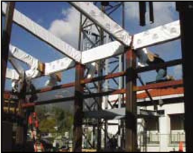
Construction activity at Los Angeles Mission College's Addition to the Instructional Student Services Building. A ribbon cutting to celebrate the completed project took place in October.
