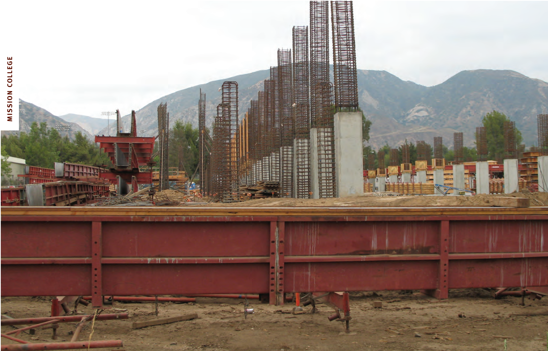
To prepare for growth at Mission College, a new parking structure is under construction. Slated for completion in March 2007, it will contain 1,200 parking spaces and will feature photovoltaic cell arrays on the roof.
