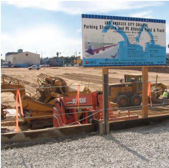
TOP: New entrance monument CENTER: Rendering of new Satellite Campus incorporating former Van de Kamp Bakery building BOTTOM: New parking lot /athletic facility under construction
